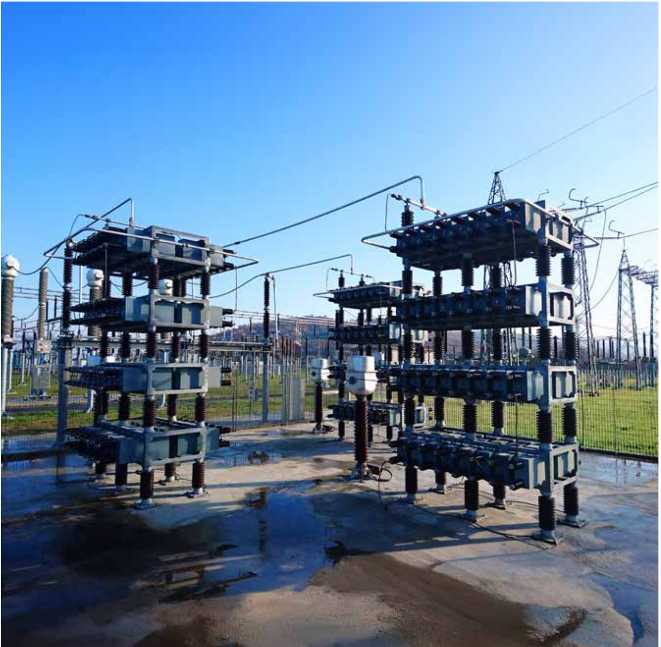
Fig. 24: Capacitor Bank 80 Mvar, 220 kV
