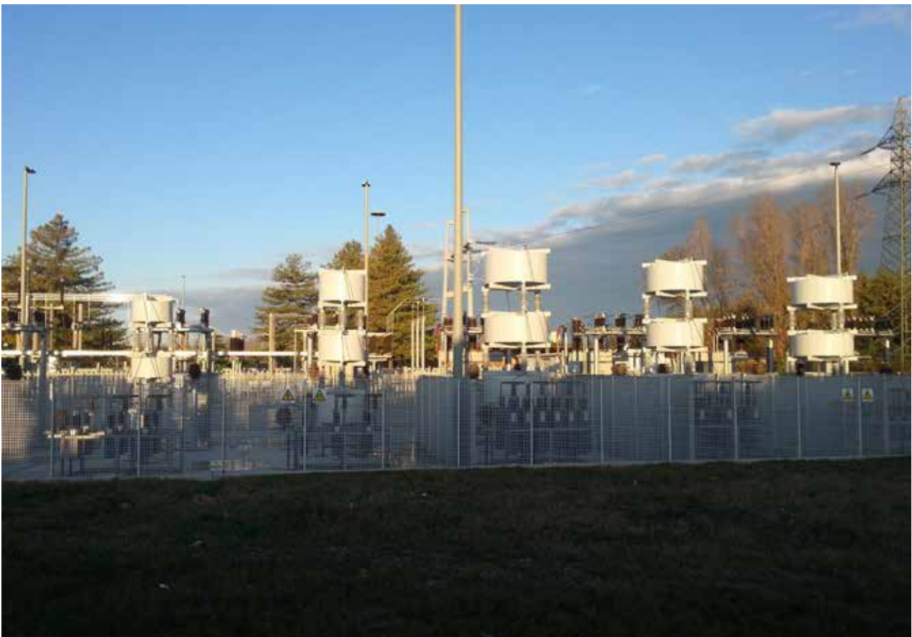
Fig. 46: System filters 24 kV
