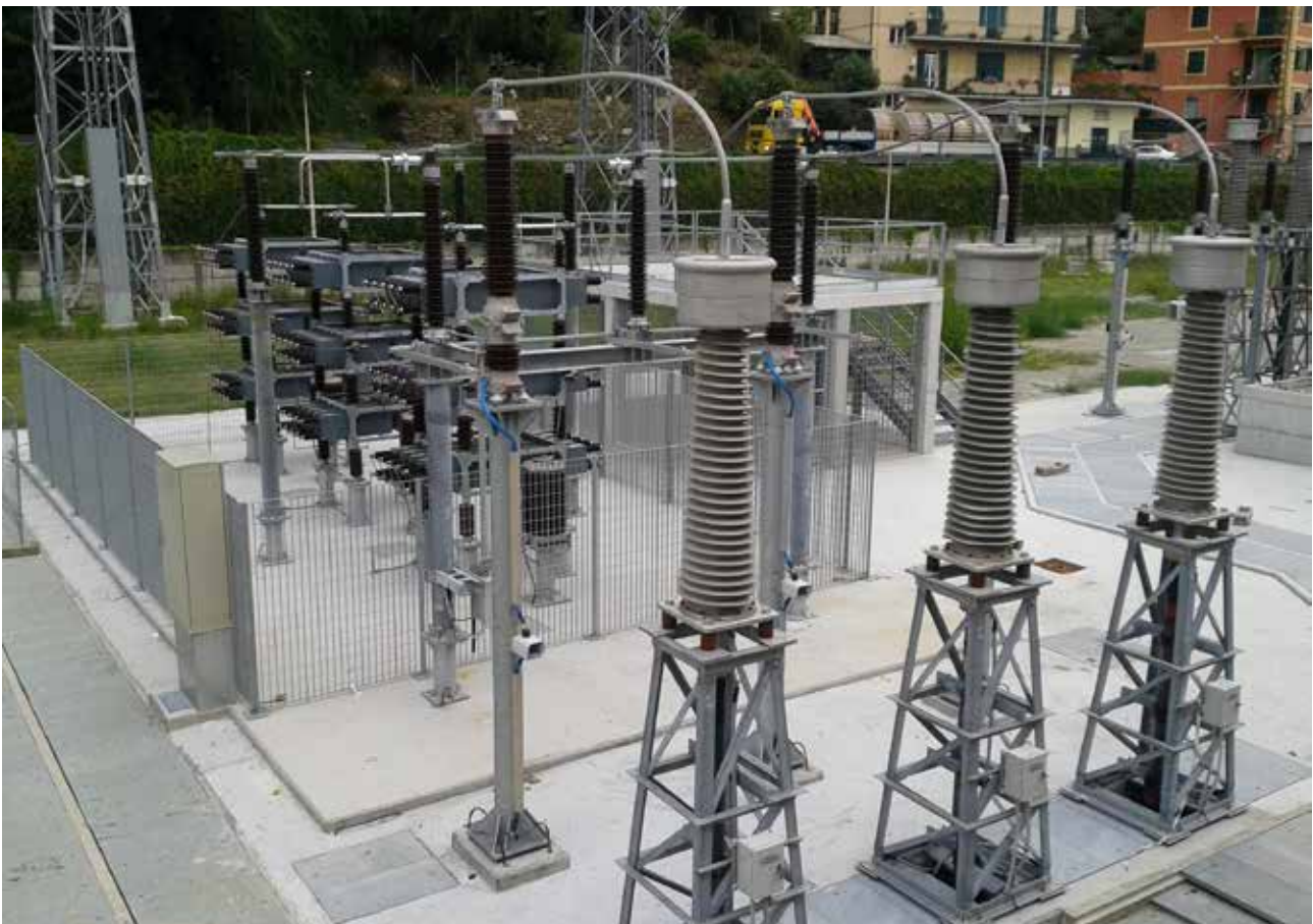
Fig. 34: 132 kV, 54 Mvar Capacitor Bank
